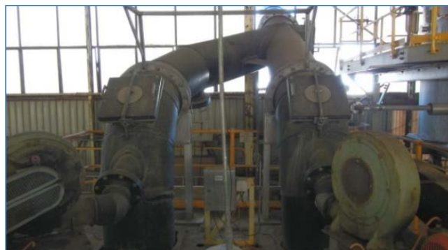
Image 1: Purification tank extraction system (Roseberg 2015)
